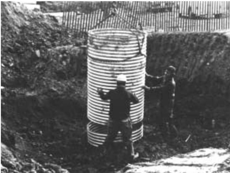
Saddle branch manhole is bolted to sewer conduit while riser extension is being lowered and coupled.
