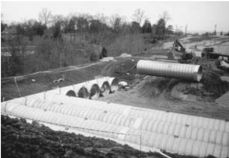
Manifold system used for underground detention.
