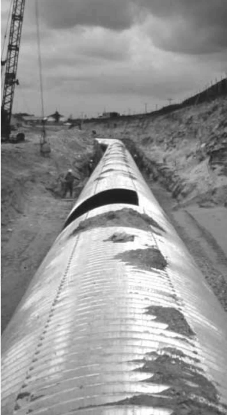
CSP sewer designed for very wide trenches.
