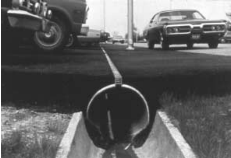
CSP concrete-lined pipe.
